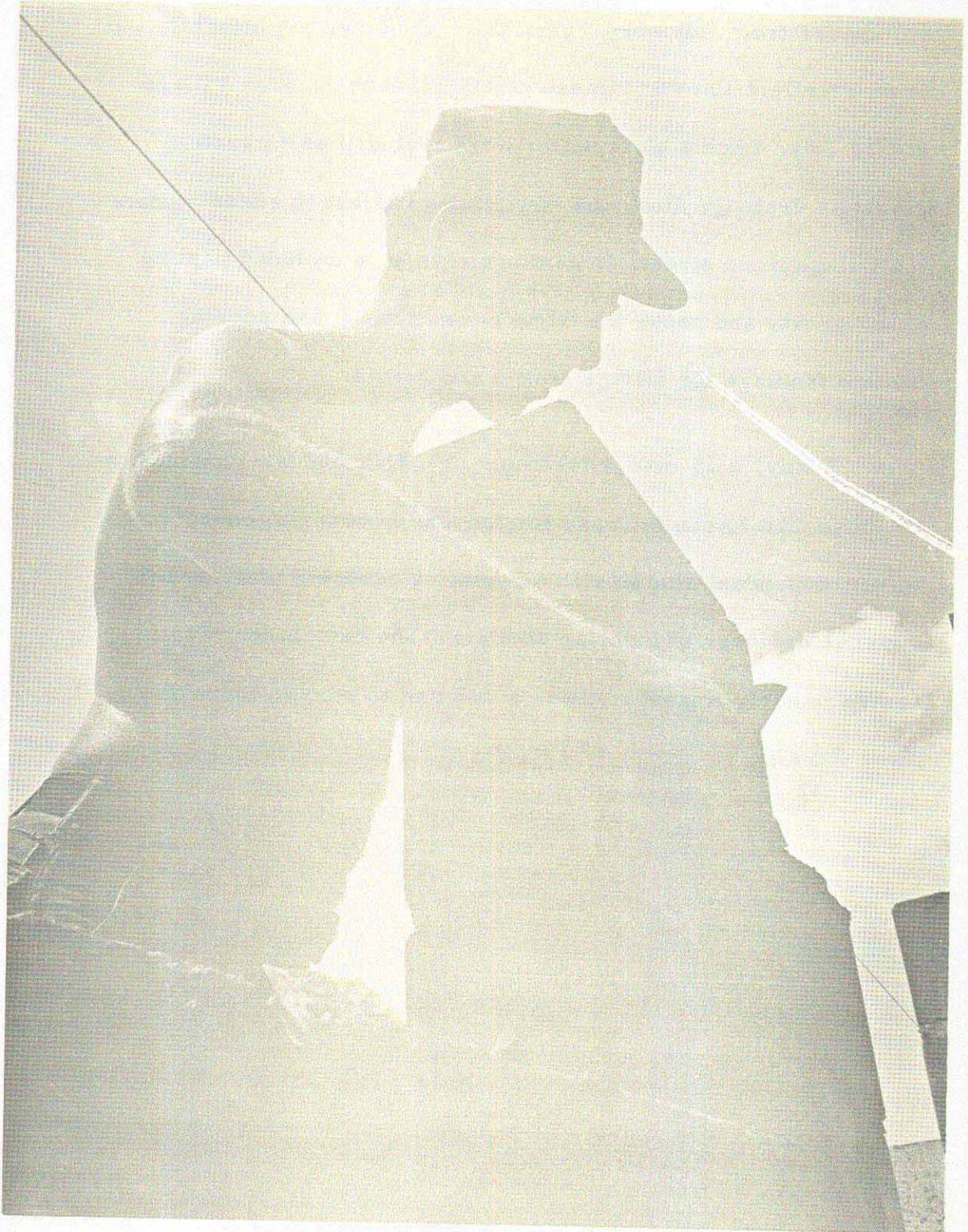
Petty Officer Third Class John B. Moran, a Navy Seabee, puts his masonry skills to work on a dependent shelter project at Cat Lai.
